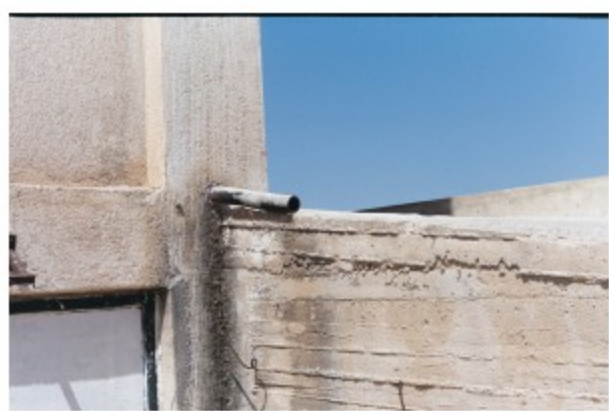
above: pipework coming out of wall, part of some sort of storage somewhere outside Lavrio, Attica district
